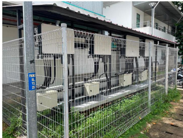
Figure 1. Solar power inverter.
